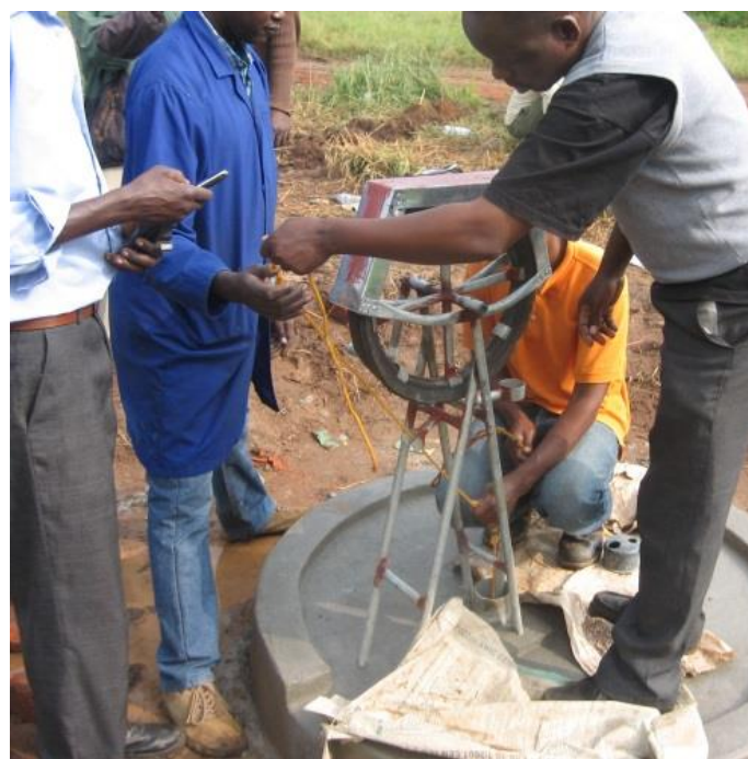
Figure 21: Installing Rope Pump during World Vision Self-supply Training, Gulu in July 2012 (Photo: Jake Carpenter)
