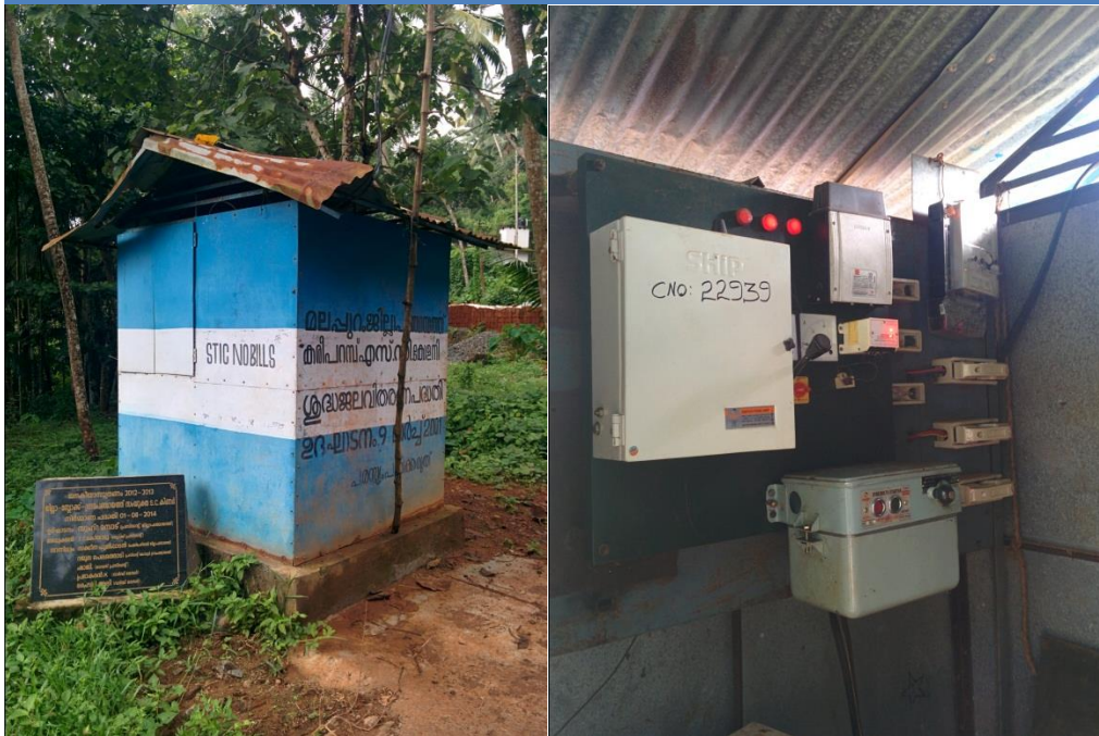
Photographs 4&5: Pump house of the Keriparambu scheme
