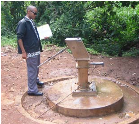
A Hand Pump Mechanic examines a faulty Shallow Well in Kisomoro Sub County, Kabarole District
