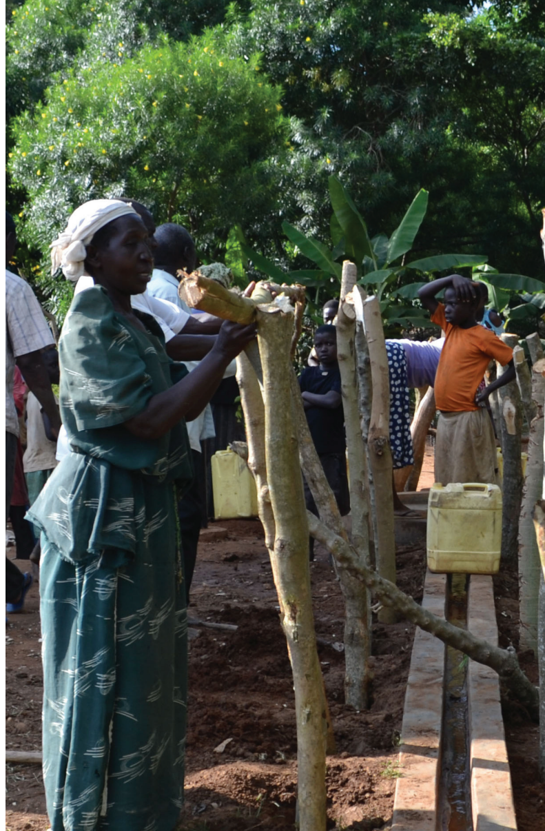
Residents of Kayinja Village, Kasodo Sub County, Pallisa district, erect a new fence around their borehole. The old fence was vandalised by people who want to use the poles for firewood. Photo UWASNET/Rehema Aanyu
