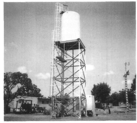
Yirimadio's Simplified Water System: A well with an electric pump feeds a raised water storage tank, which provides water to three standpipes.
