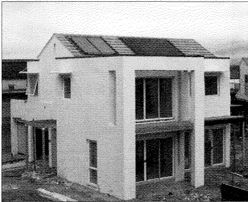
Figure 2 Typical house in solar village showing hot water system and PV on roof
