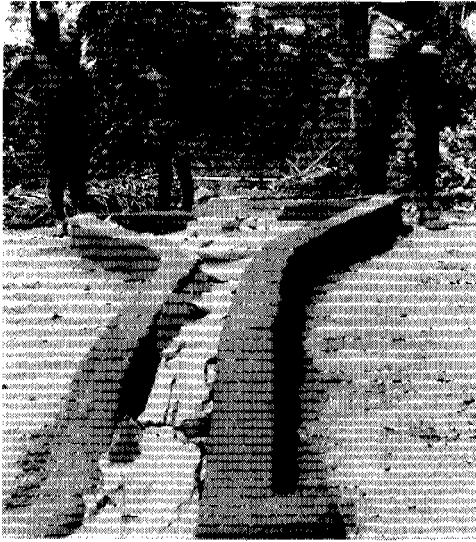
Figure 6.6 Use of moist sand or leaves is a more effective way of curing the concrete than these dry sacks. Keeping the concrete moist for several days is essential for proper curing
