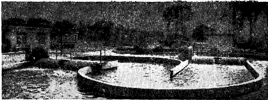
Effluent Treatment Plant at Hindustan Machine Tools Ltd., Bangalore.
