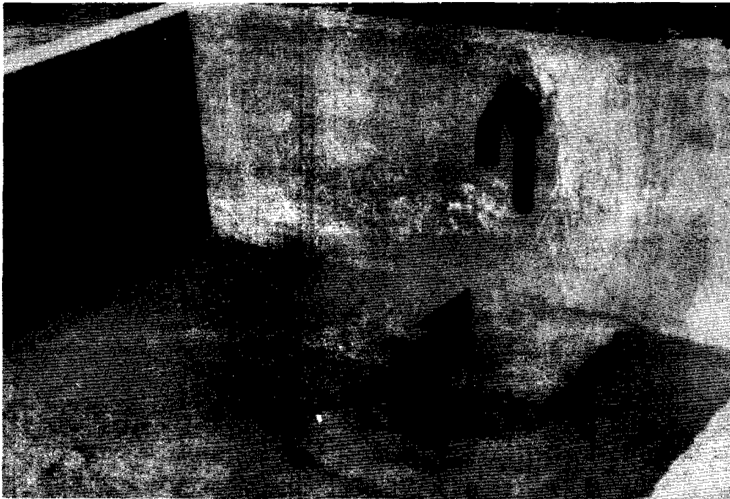
The slow sand filter showing inlet cum drain out chamber
