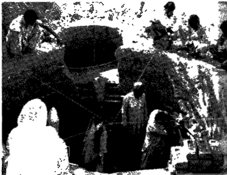
Interested spectators watch the construction of the impermeable brick lining for the bio-gas tank.
