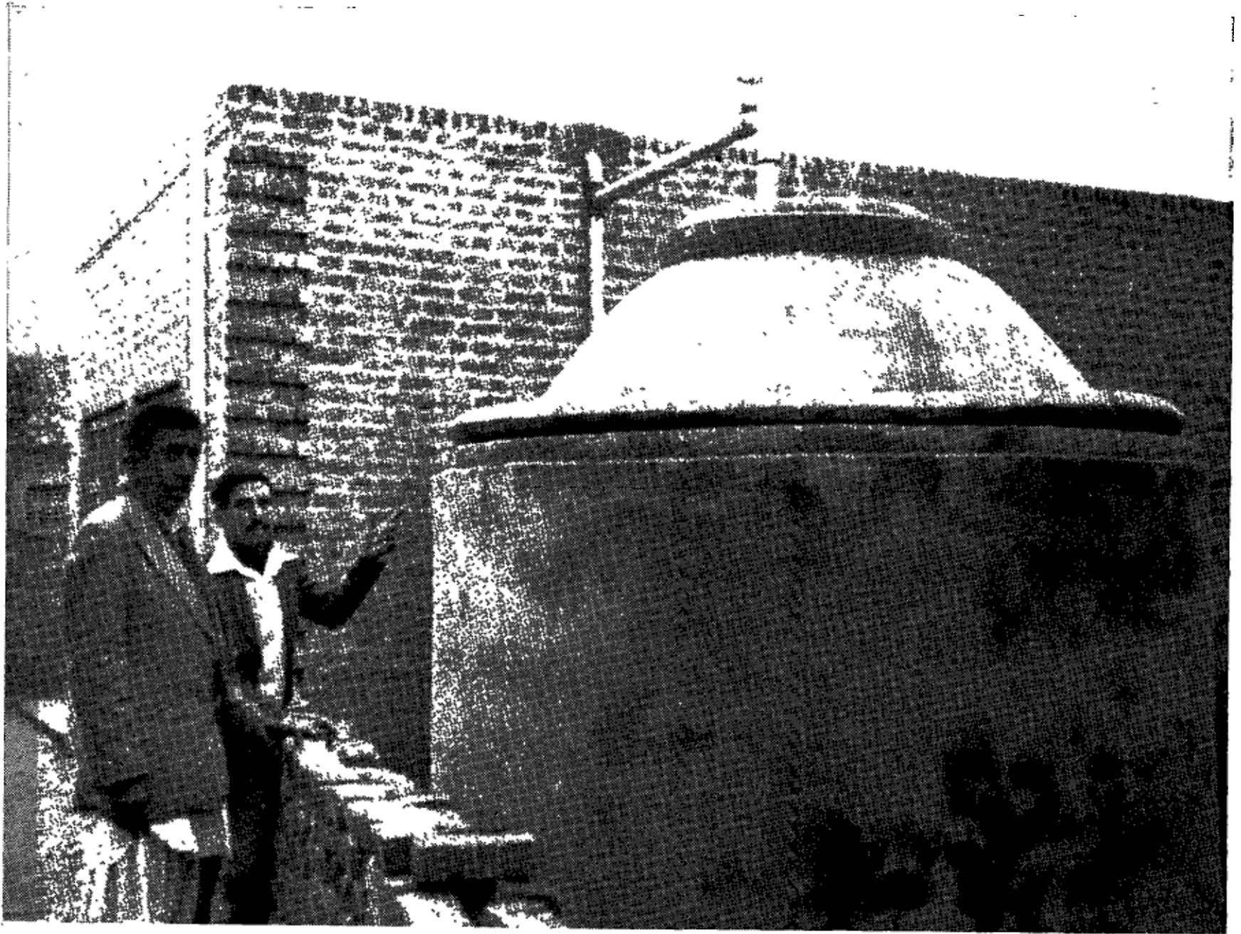
A complete water cistern showing the pipes which channel water from the roof of the house into the tank.
