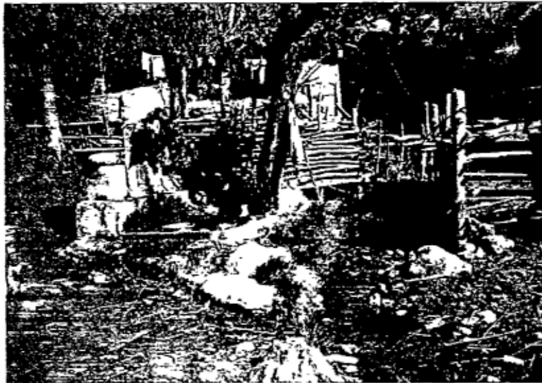
Tapstand with dirty surrounding
