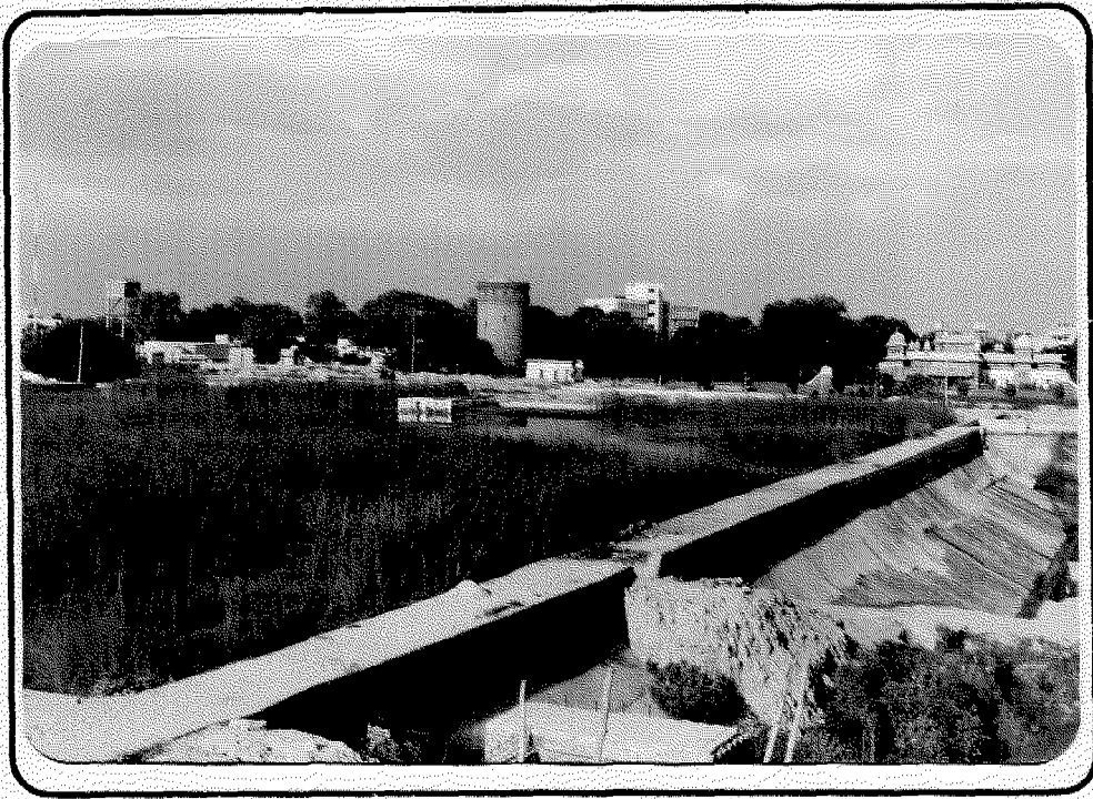
SILTED SEDIMENTATION TANKS AND AQUATIC WEED GROWTH RESULT OF NEGLECTED MAINTENANCE
