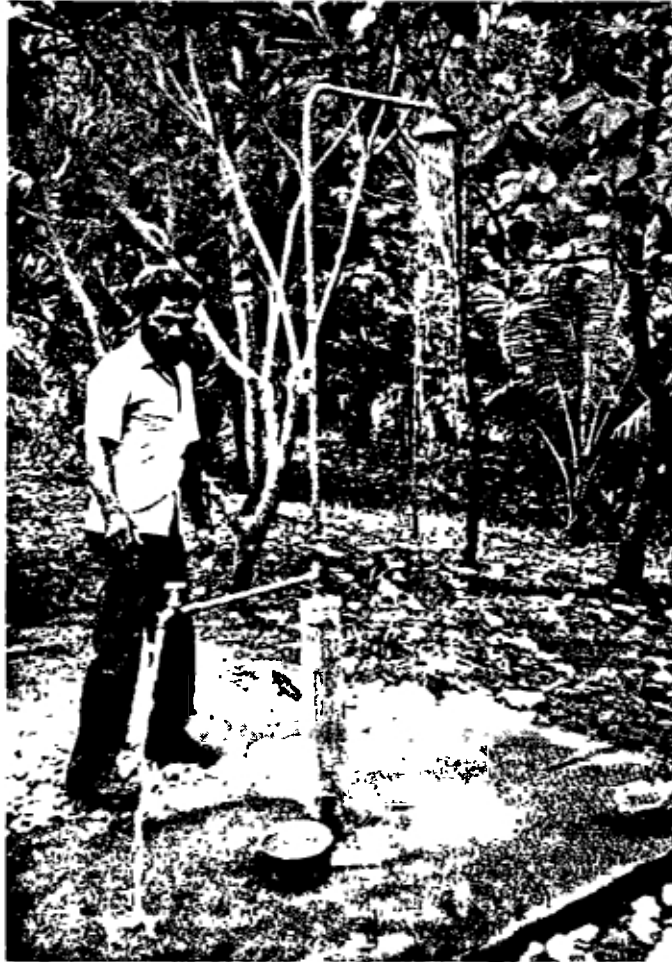
27. Public tap and shower installation.
