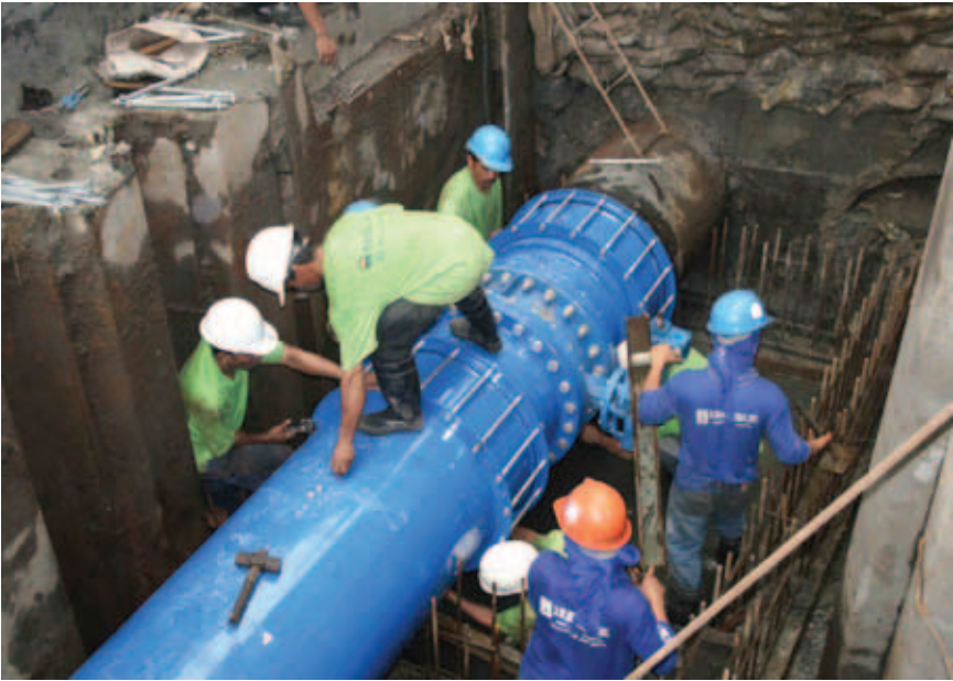
Maynilad contractors at work during an interconnection activity in Sta. Mesa, Manila. Photograph courtesy of Federico Juane, Maynilad Water Services.
