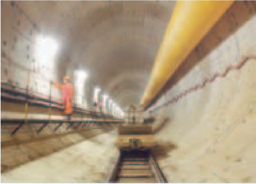
A tunnel of the Deep Tunnel Sewerage System: The system was conceived as a long-term solution to meet Singapore's needs for used water collection, treatment, and disposal through the 21st century. Photograph courtesy of the Public Utilities Board.
