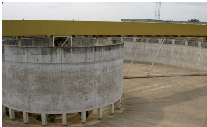
Settlement Tank, Cross River State, Nigeria
