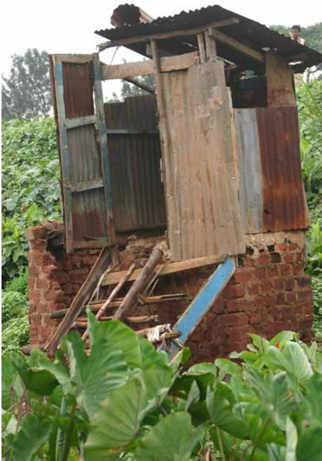
Inaccessible latrine for mobility impaired
