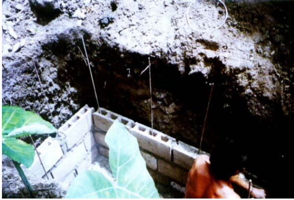
Construction of leaching pit for pour flush toilet using hollow blocks, Barangay 15
