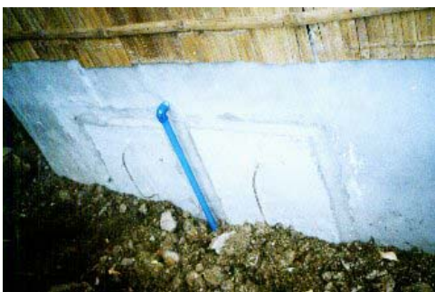
Back of toilet unit - access doors to vaults and drain of cleaning basin
