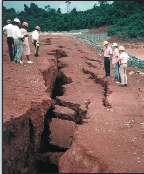
Officials inspect a giant crack at the MIGA-insured Omai gold mine in Guyana. In 1995, a tailings dam broke at the mine, spilling billions of liters of cyanide-laced effluent into a local river. (Photo: Mineral Policy Center)
