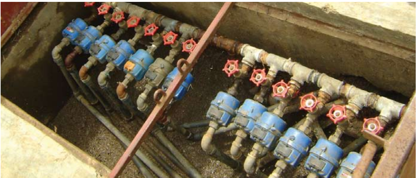
Meter chamber on Line 1
