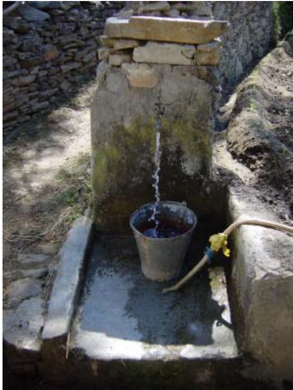
Pipeline for domestic water supply, India
