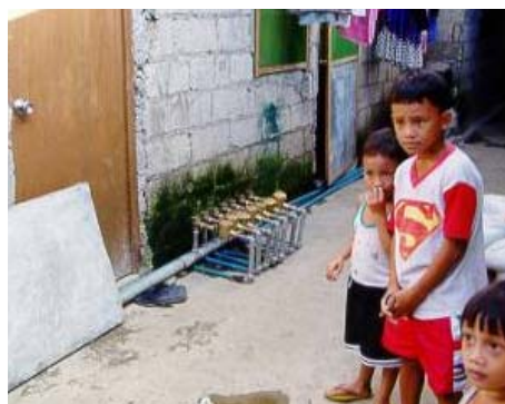
Photo 4 – Meter battery in a Manila street (Photo Maynilad)
