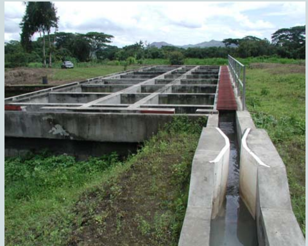
Flow measurement (Parshall channel) and Imhoff tank at the SSHF constructed scheme at Masatepe, Nicaragua. Source: Martin Gauss, 2005.
