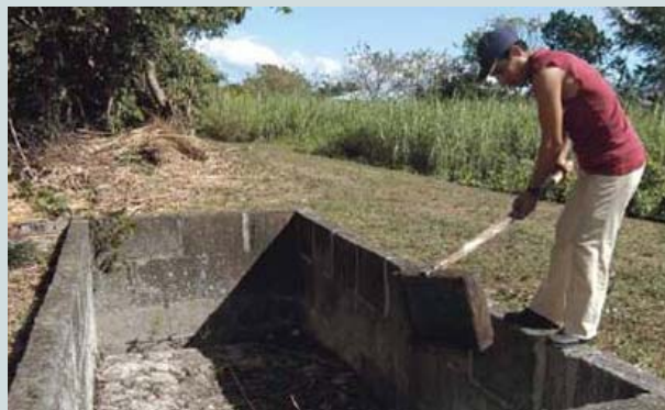
Operator discharging sludge from the grit tank to the drying bed. Source: WSP, 2006.
