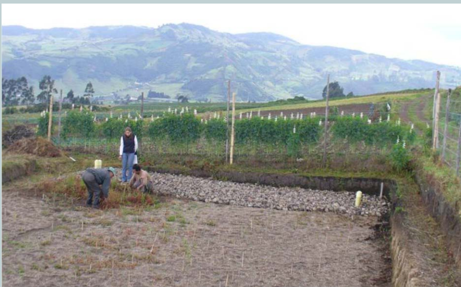
SSHF constructed wetland in Pasto, Colombia, during construction. Source: K. Moncayo, personal communication, 2007.
