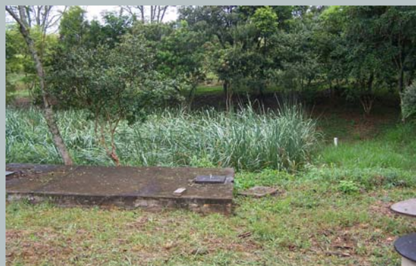
Septic tank and constructed wetland installed at EPAGRI at Florianópolis, Santa Catarina, Brazil. Source: WSP (2007).
