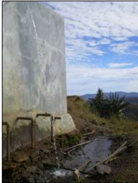
Figure 5 Storage tank in Taiblolor community built three years previously, Aileu District.
