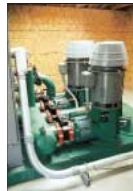
This set of variable frequency drive pumps allows maximum flexibility in irrigating the entire course in the shortest period of time, improving efficiency and reducing energy cost.
