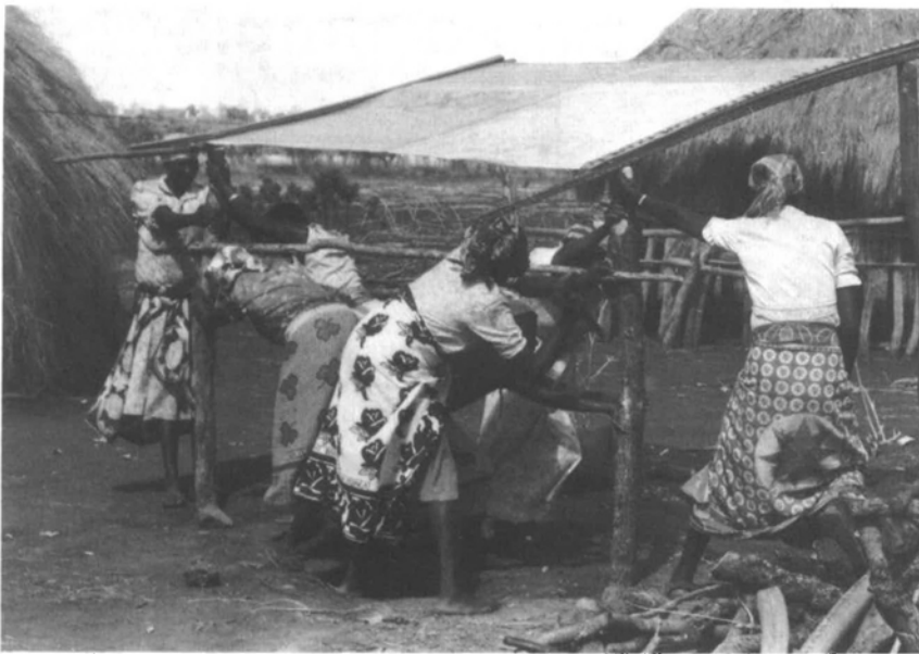
The sheet is nailed to two poles and then mounted on four upright poles.
