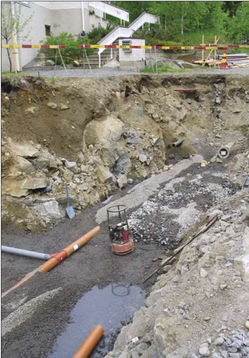
In Finland it is common practice to lay pipes for water and wastewater utility services in the same trench, which reduces the disruption to the public as well as costs in terms of excavation and labor.
