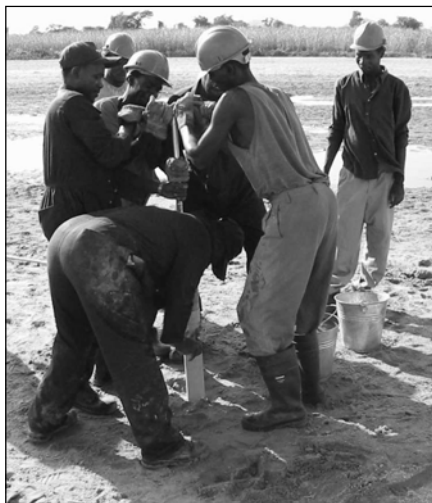
The bailer and stem are withdrawn while the casing is pushed further into the ground.
