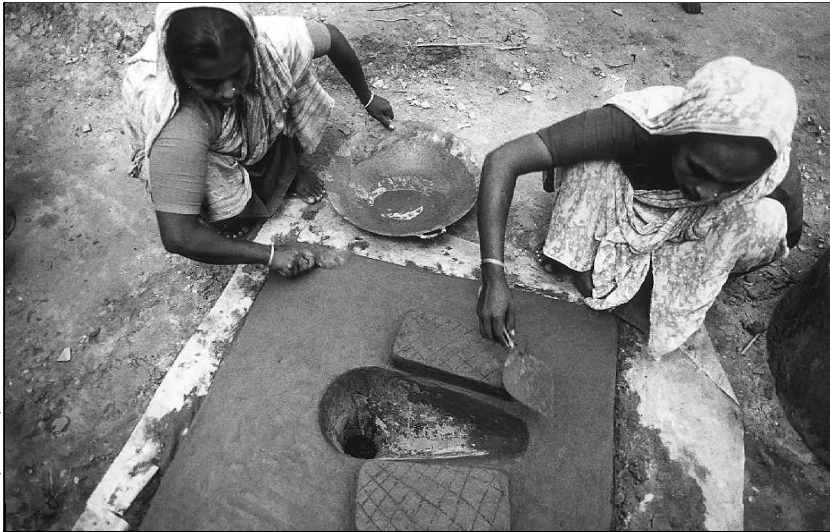
Women finish work on a latrine. On-site sanitation is likely to be the major source of chemical contamination in the study areas.
