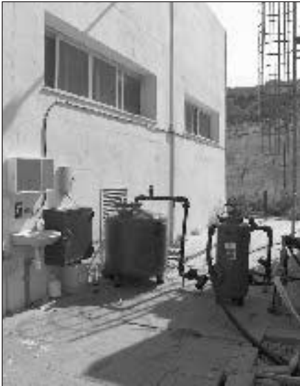
The disinfection system rendered the reclaimed water suitable for unrestricted irrigation
