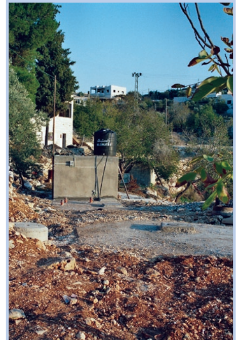
Photo 5-8: Greywater treatment plant in Al-Zaitunah, Palestine (photo: Sandec)
