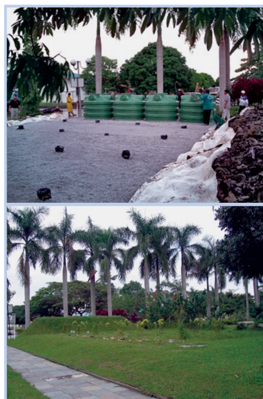
Photo 5-9: Aerobic filters and planted filter under construction (top) and completed (bottom) in Hui Sing Garden, Kuching (photo: NREB, 2003, Martin C., 2005)
