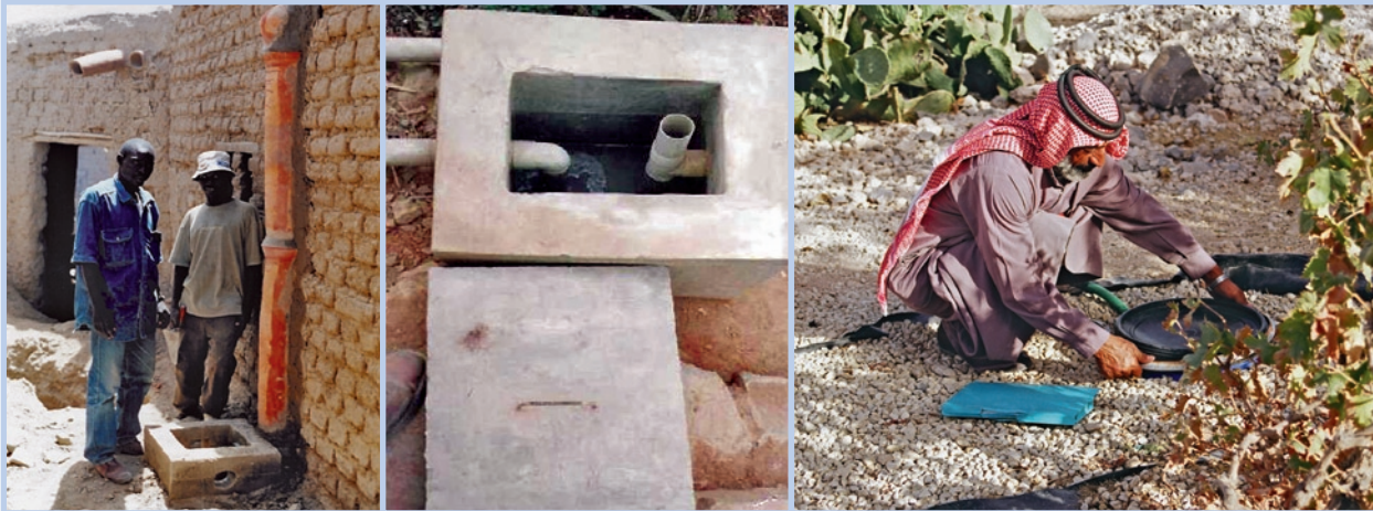
Photo 4-4: Left: Grease and grit trap used as primary treatment unit in a greywater infiltration system in Djenné, Mali. Given its small size, the trap often clogs, thus jeopardising the subsequent infiltration system (photo: Alderlieste M.) Centre: Grease trap implemented in a household greywater irrigation system in Peru. The trap is undersized, vertical baffles are missing, resulting in clogging of the subsequent planted filter (photo: García O.) Right: Buried, recycled 160-litre plastic barrel used as grease trap and grit chamber ahead of an unplanted horizontal-flow gravel filter in Jordan (photo: Kassay J., IDRC)
