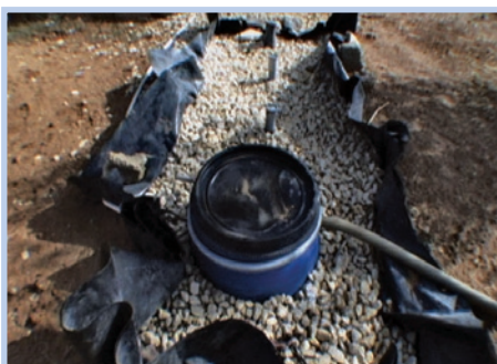
Photo 5-7: Horizontal-flow filter and storage tank (photo: Ghose R.)
