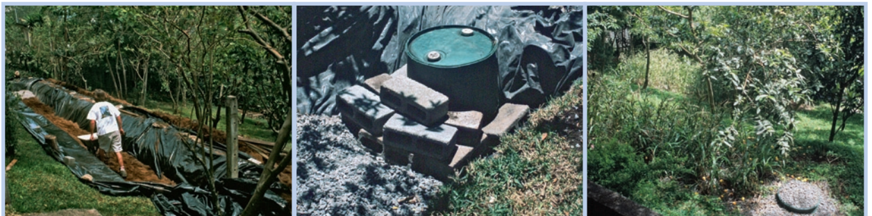
Photo 5-5: Build up of 1 st reedbed: Excavation (left), inlet drum (centre) and planted filter (right) (photos: Dallas S.)
