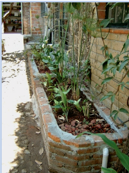
Photo 4-6: Horizontal-flow planted filter treating greywater of one household in Tepozlán, Mexico (photo: Sandec)
