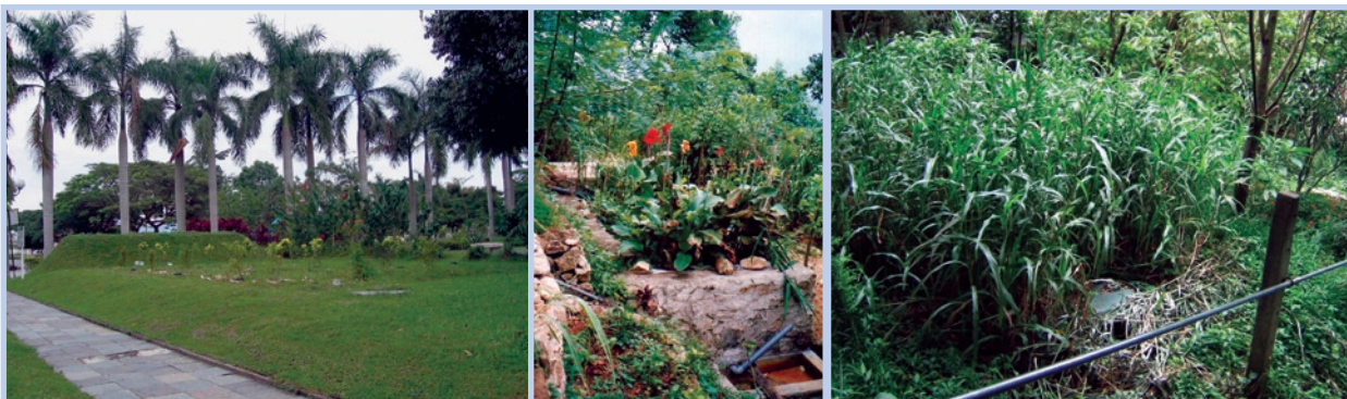
Photo 4-8: Left: Subsurface horizontal-flow filter (crushed limestone) fed by pretreated greywater from a neighbourhood of 45 persons in Kuching, Sarawak, Malaysia. The vegetation has an ornamental function only. The filter surface amounts to 2.8 m 2 per person equivalent (photo: Martin C.)
