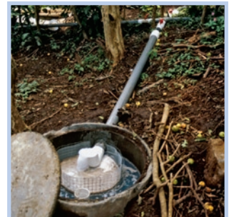
Photo 5-4: Settling tank (photo: Dallas S.)
