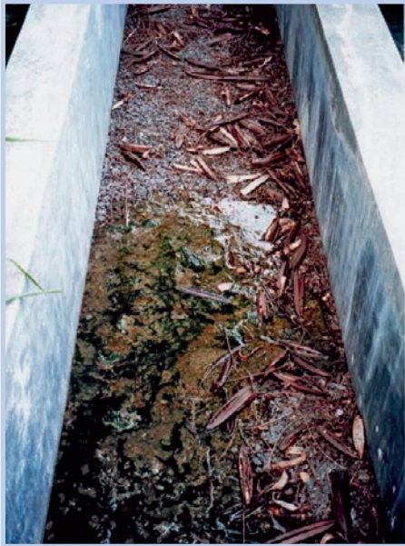
Photo 4-7: Clogging of the inlet zone of an unplanted horizontal-flow filter, indicating an overload of the inlet zone, possibly caused by the high L:W ratio, Sri Lanka (photo: Harindra Corea, E.J.)
