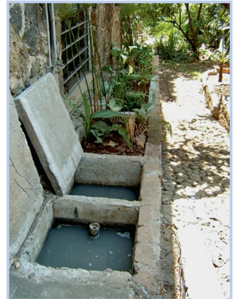
Photo 4-3: Grease trap ahead of horizontal-flow planted filter installed in Tepoztlán, Mexico (photo: Sandec)
