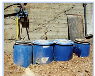
Photo 4-5: Four-barrel up-flow anaerobic filter implemented in Jordan. Two tanks of 220-litre capacity each filled with gravel media acting as anaerobic filters are inserted between a sedimentation and a final storage tank (photo: Redwood M., IDRC)
