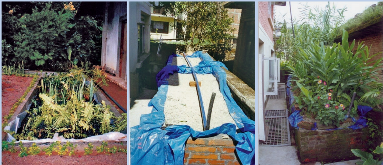
Photo 4-9: Left: VFPP treating kitchen and laundry greywater in a hotel in Sri Lanka, after pretreatment in a grease trap and septic tank (photo: Harindra Corea E.J.)
