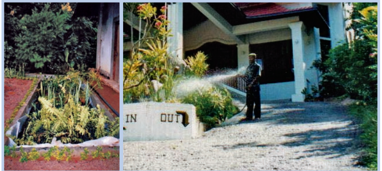
Photo 5-10: VFPP for greywater treatment at Swiss Residence Hotel in Kandy (left). The treated effluent is reused for gardening (right) (photo: Harindra Corea E.J.)
