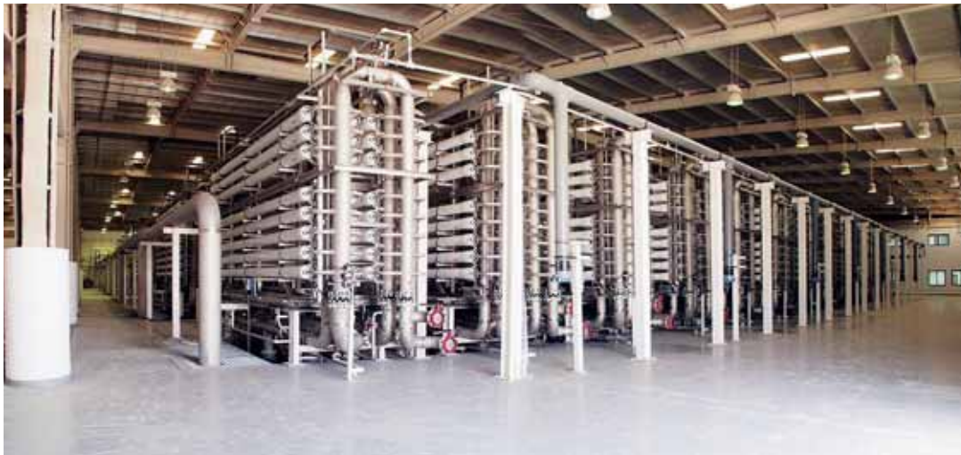
Completed in 2004, the Sulaibiya Wastewater Treatment plant in Kuwait is one of the largest of its kind in the world (Source: Norit)
