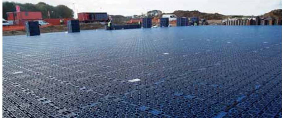
Collect and store: Wavin solutions in practice. To minimise the risk of flooding in the area, this substantial underground storage facility with AquaCell units was created. The structure can cope with the drainage requirements of 1,500 houses!
