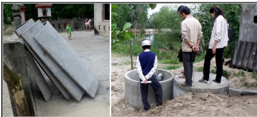
Figure 4.6 – Steel moulds of concrete rings and demonstration septic tanks in Trieu An commune
