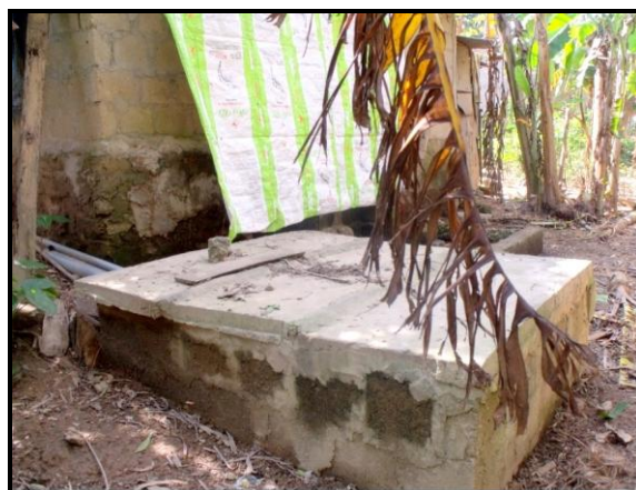
Figure 4.4 - Septic tank in the garden in Trieu Do commune
