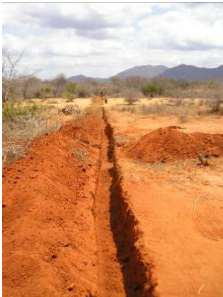
157 km of trenches were excavated and pipes laid in the trenches and back-filled for the 6 water projects.
