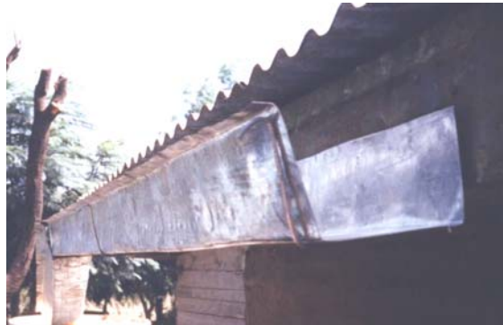
Square gutter fixed without splash-guard.
