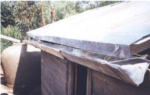
V-shaped gutter suspended from a splash-guard.
