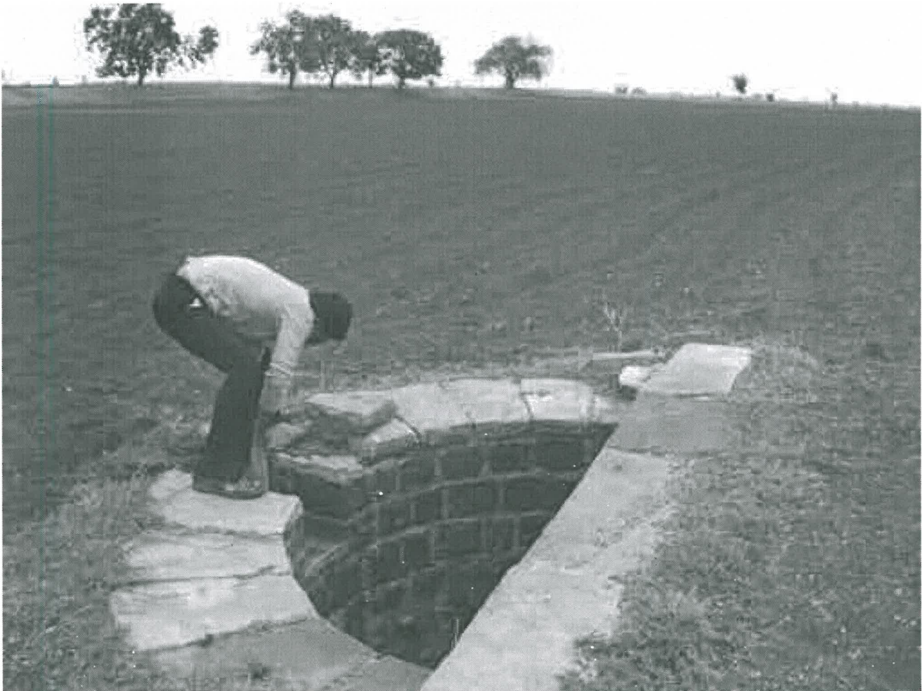
A concealed spillway in one of Mallanna's Ramavadagi fields. A single stone can control the run-off. Uneven and infertile a century ago, this field is as fertile as any other in the area.
