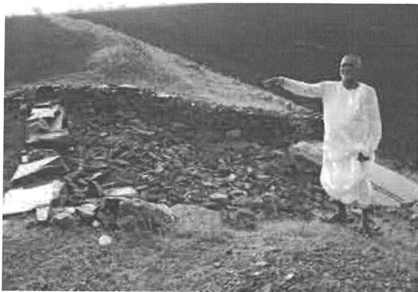
Dr Mallanna near a simple open spill-way, explaining its principle. For small fields the open spillway is sufficient.
