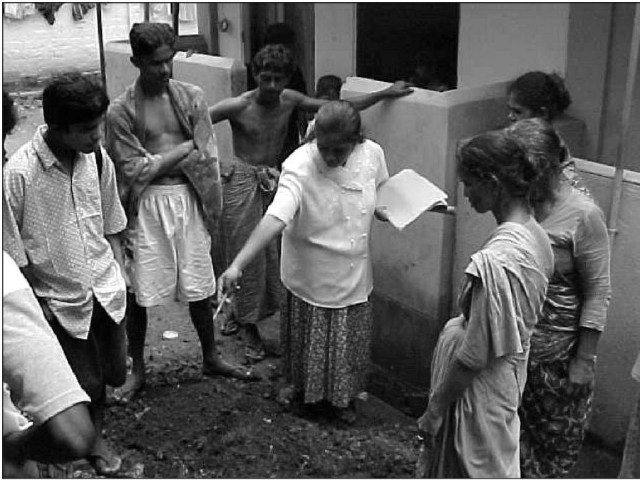
The work is discussed on site. To bring connection costs down householders themselves dig the trench and backfill it when the pipe is laid
