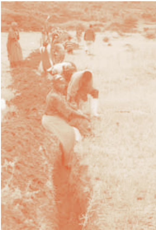
Community members in Ngedlengedle in KwaZulu-Natal province work together to dig trenches for their water supply system
