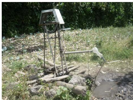
Figure 3-9 Poorly installed rope pump, Meskan
