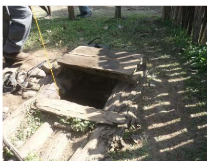
Figure 3-7 Wooden support with lid, Meskan
