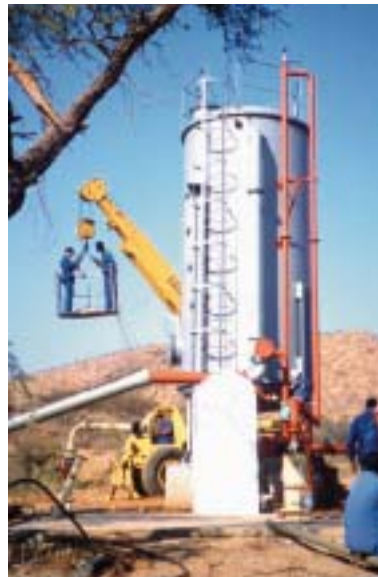
Figure 5. Activated carbon filter, Windhoek (Murray & Tredoux, 2002b).
