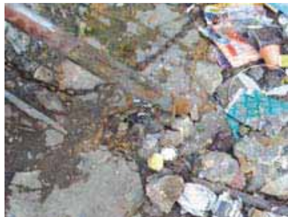
Partially exposed networks in Hay el Sohoun cause potential water contamination by sewage
