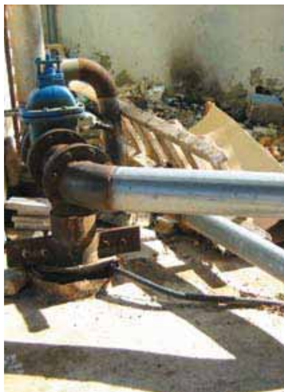
Water well established by PLO for water provision in Ain el Helwe Camp and Fadlo Wakim
