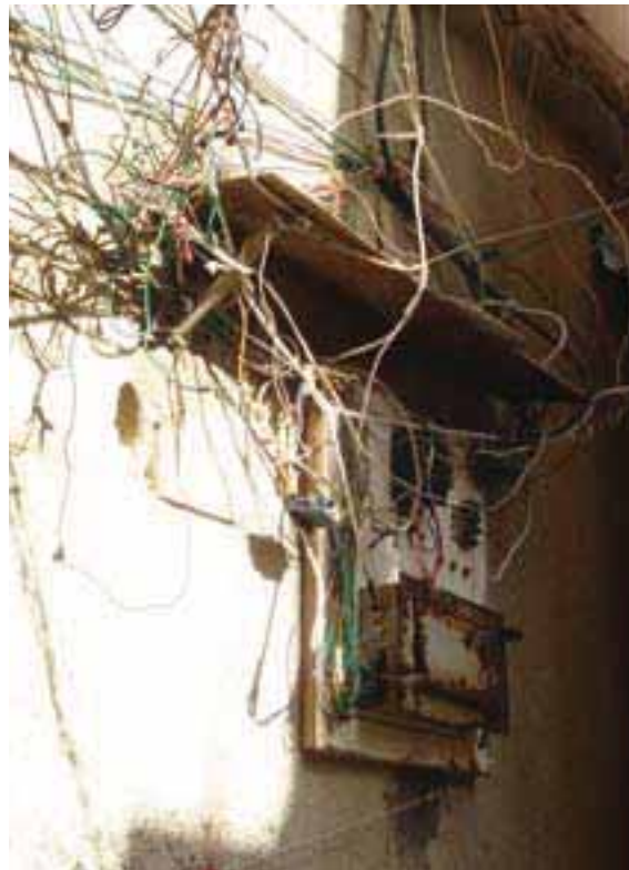
Unorganized electricity connections from a distribution board in Bustan el Kods
