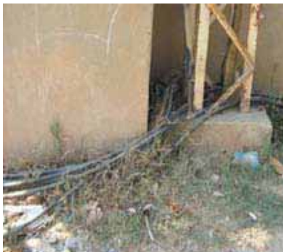
Water reaches houses through above-ground plastic networks installed by dwellers in Tallet el Mankoubin
