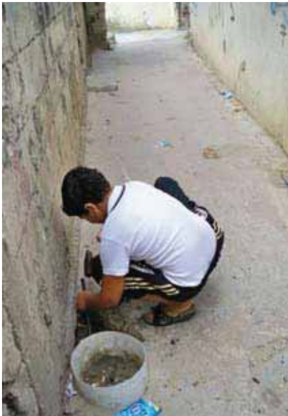
A young dweller resorting to unblocking sewage congestion by manually breaking manholes
