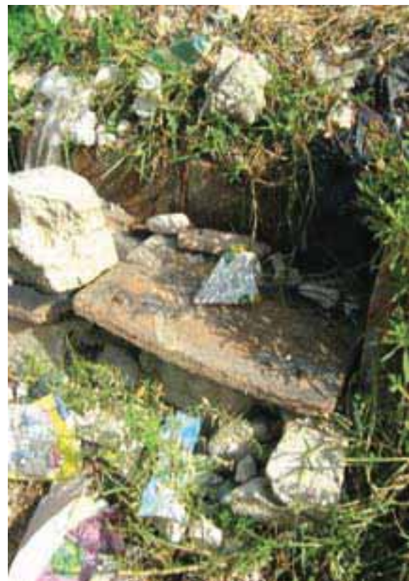
Exposed septic tanks in Jabal el Halib
