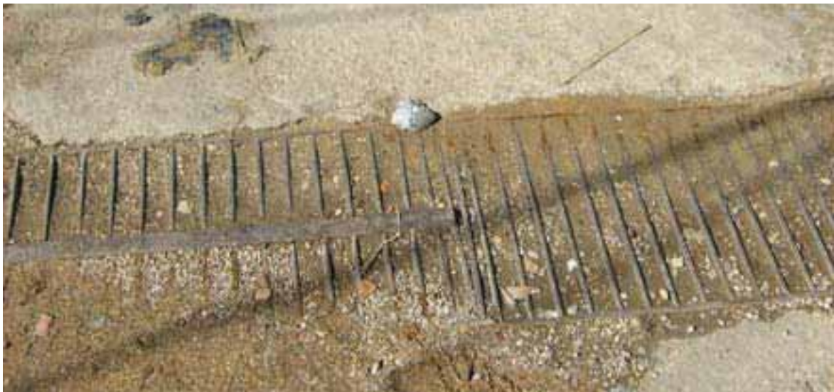
One water drain (blocked) was installed by UNRWA at the entrance to Fadlo Wakim
