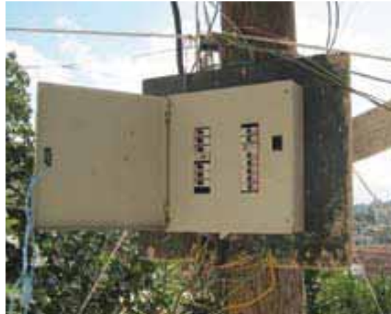
Electric distribution board installed by the Camp PC to organize electricity provision in Mieh Mieh AA
