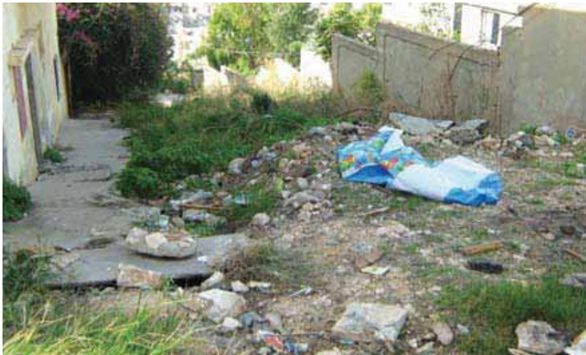
In addition to rehabilitation, roads in Jabal el Halib need a drainage system that suits the strong sloping of the AA
