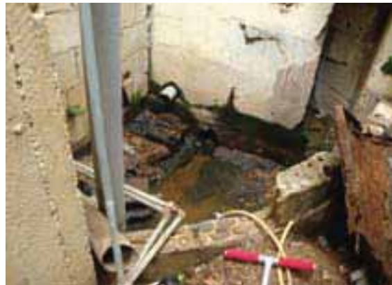
An example of water and sewage connections in Sekke
