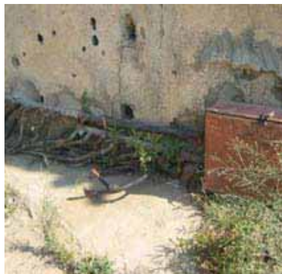
One collective manifold installed by UNICEF at the entrance of Tallet el Mankoubin provides water to all houses in the AA
