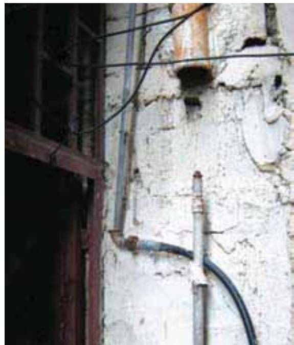
Sewage drainage and water connection methods in Tawari
