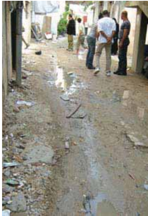
Roads in the AAs are in massive need of rehabilitation and paving, Baraksat AA around Ain el Helwe Camp
