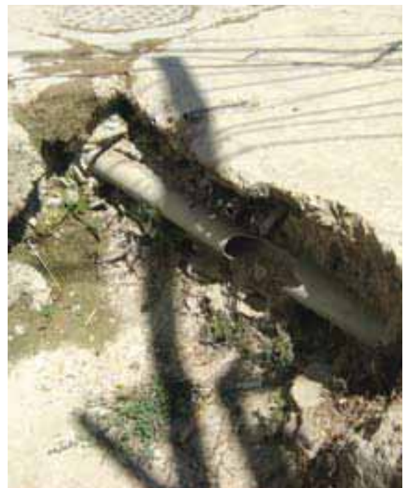
Broken sewage pipes in Mieh Mieh AA
