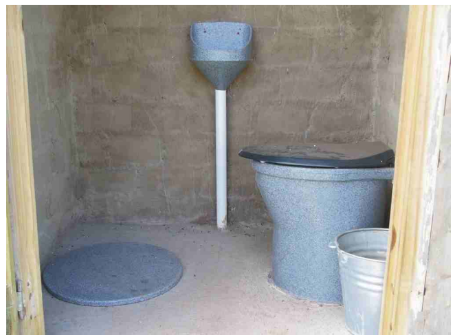
The inside of a UD toilet showing pedestal, urinal and sealed second vault
