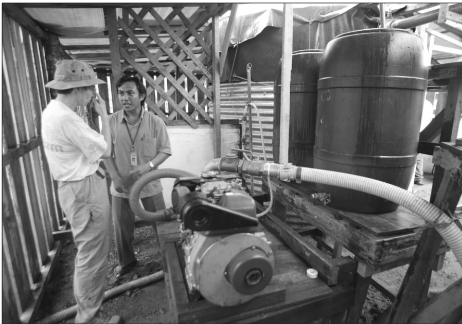
After the tsunami , there was more money so more technology: this emergency town water supply was supported by Oxfam. Credit: Jim Holmes/Oxfam
